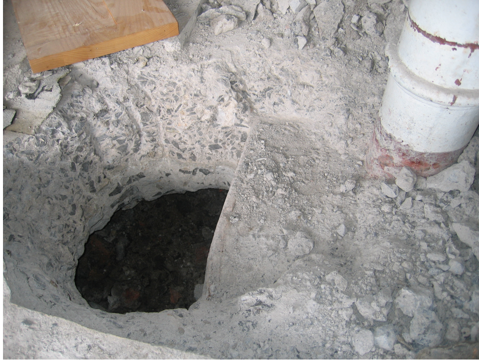
Plate 5: Trench D, located within the interior of the Barrack Coach House. The opening was cut through two levels of concrete flooring (C303 and C304) to the immediate west side of the cast-iron vehicle kerb (C306), designed to protect the cast-iron pillar (C307). The underlying foundation raft (C305) can be seen within the opened area.
