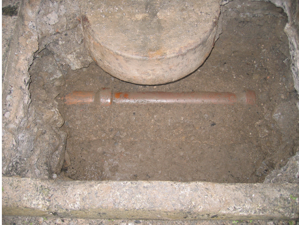
Plate 3: View of ceramic sewage pipe (C12) bedded in concrete matrix (C13) in the northern half of Trench A, with the surface of C14, a thin layer of brown clay, present in the southern sector.
