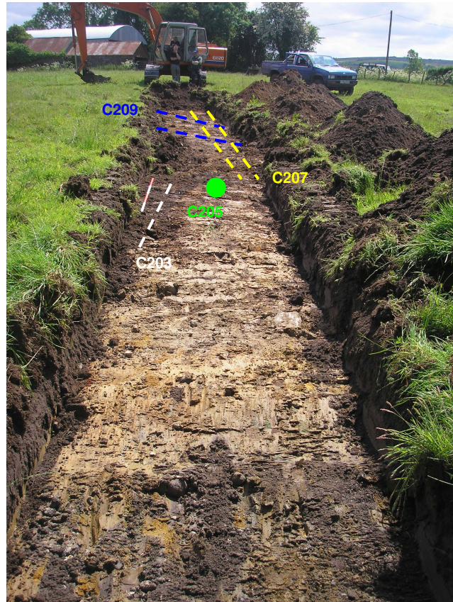
Plate Three: Annotated photograph of Trench Two following excavation to subsoil level (Context No. 211), looking south-east
