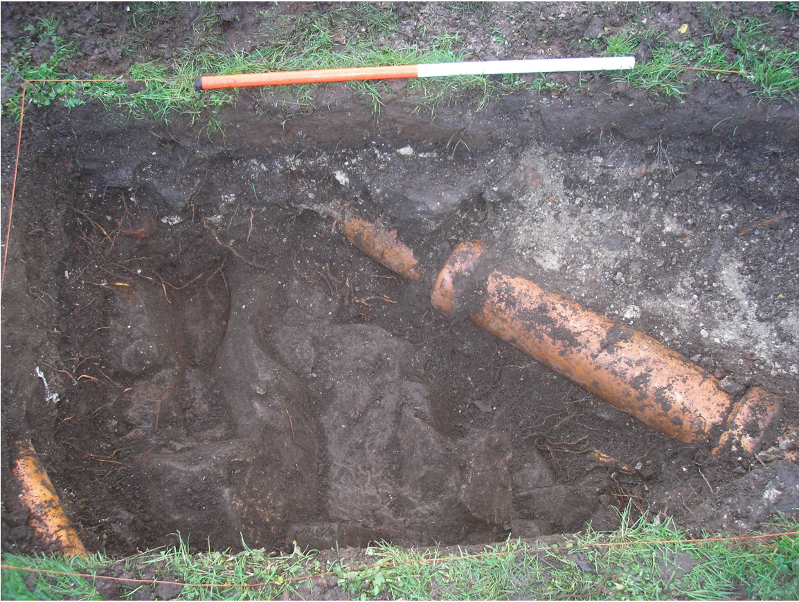
Plate 4: Trench 1 showing bedrock, service pipes and remnant mortar deposit (Context No. 104), looking east.
