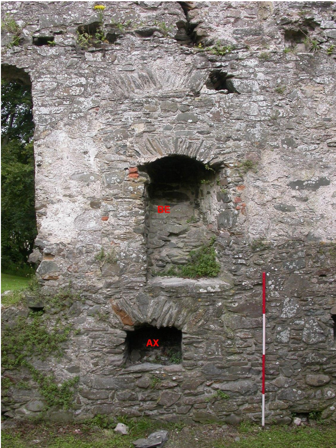
Plate 8: Part of the eastern wall of the east wing, showing internally-blocked fireplace (AX), ground-floor fireplace (BE), looking east. Also visible in the top of the photograph are the supporting holes for the crossbeams that carried the attic floor.
