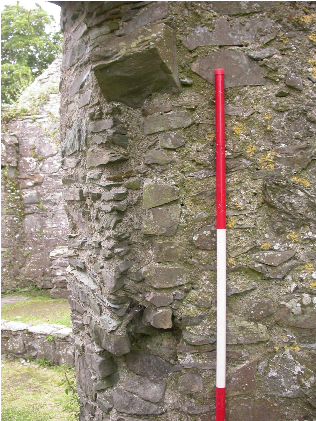
Plate 2: Surviving rebate for a wooden frame preserved in the western edge of the eastern opening in the north wall of the west wing (AC), looking southwest. Scale divisions 0.5 metres.
