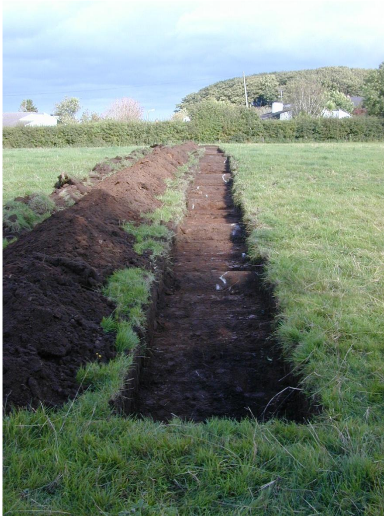
Plate 27 Trench D: mechanically excavated trench in Area 3, located approx. 14m north of Trench C (facing East).
