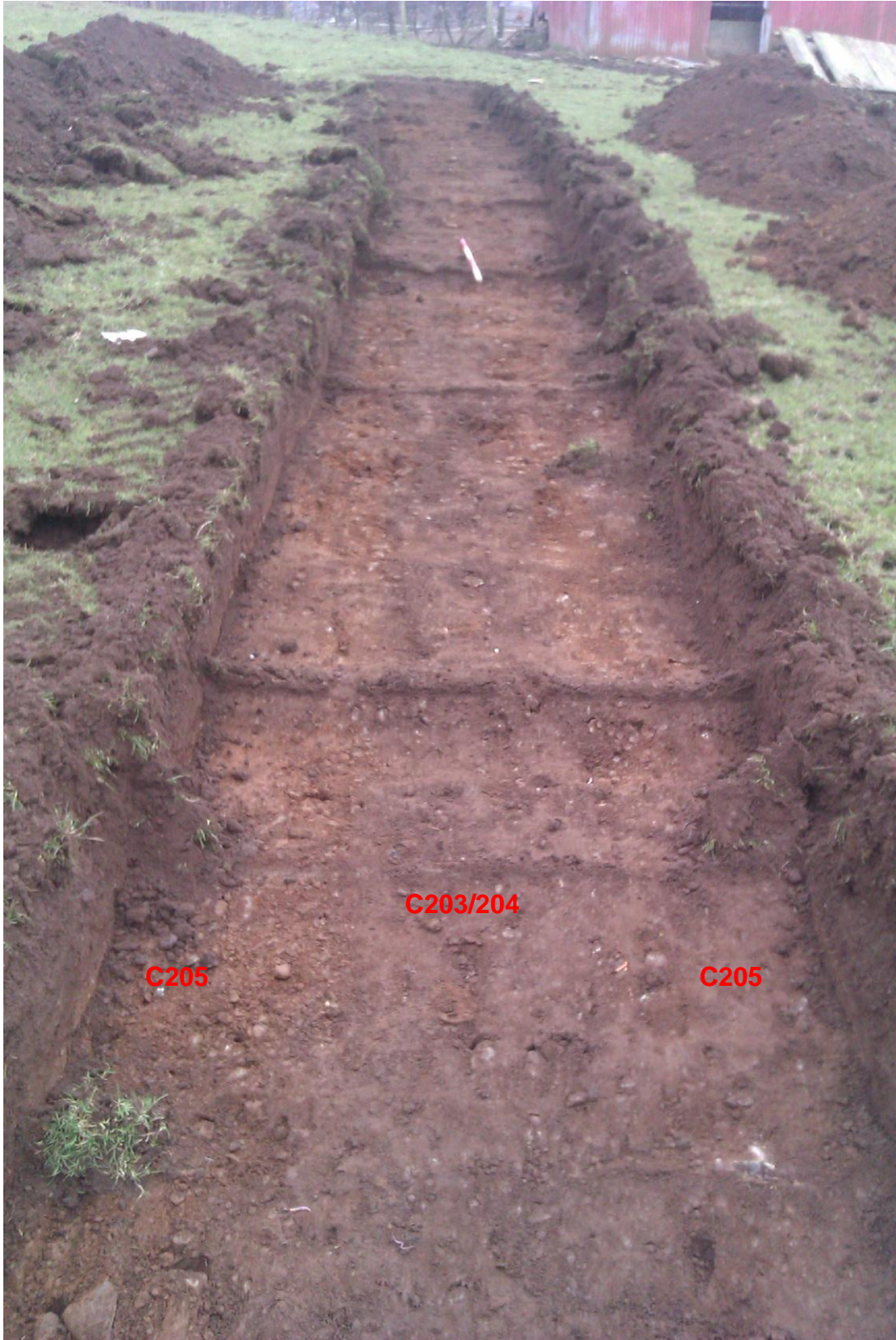
Plate 12: Trench 2 following excavation to subsoil level and showing linear feature (C203/204), looking west
