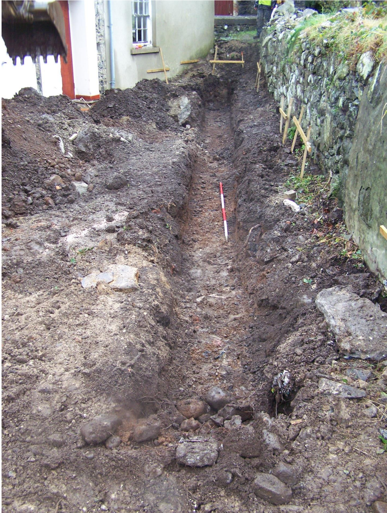
Photo 4: Area 4 showing foundation trench for east wall of kitchen block / toilet extension.
