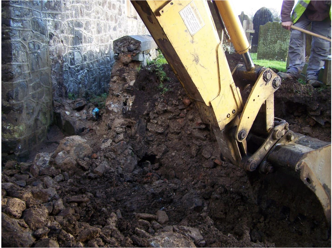
Photo 3: Removal of retaining wall (Area 3) to west of graveyard by mechanical excavator.
