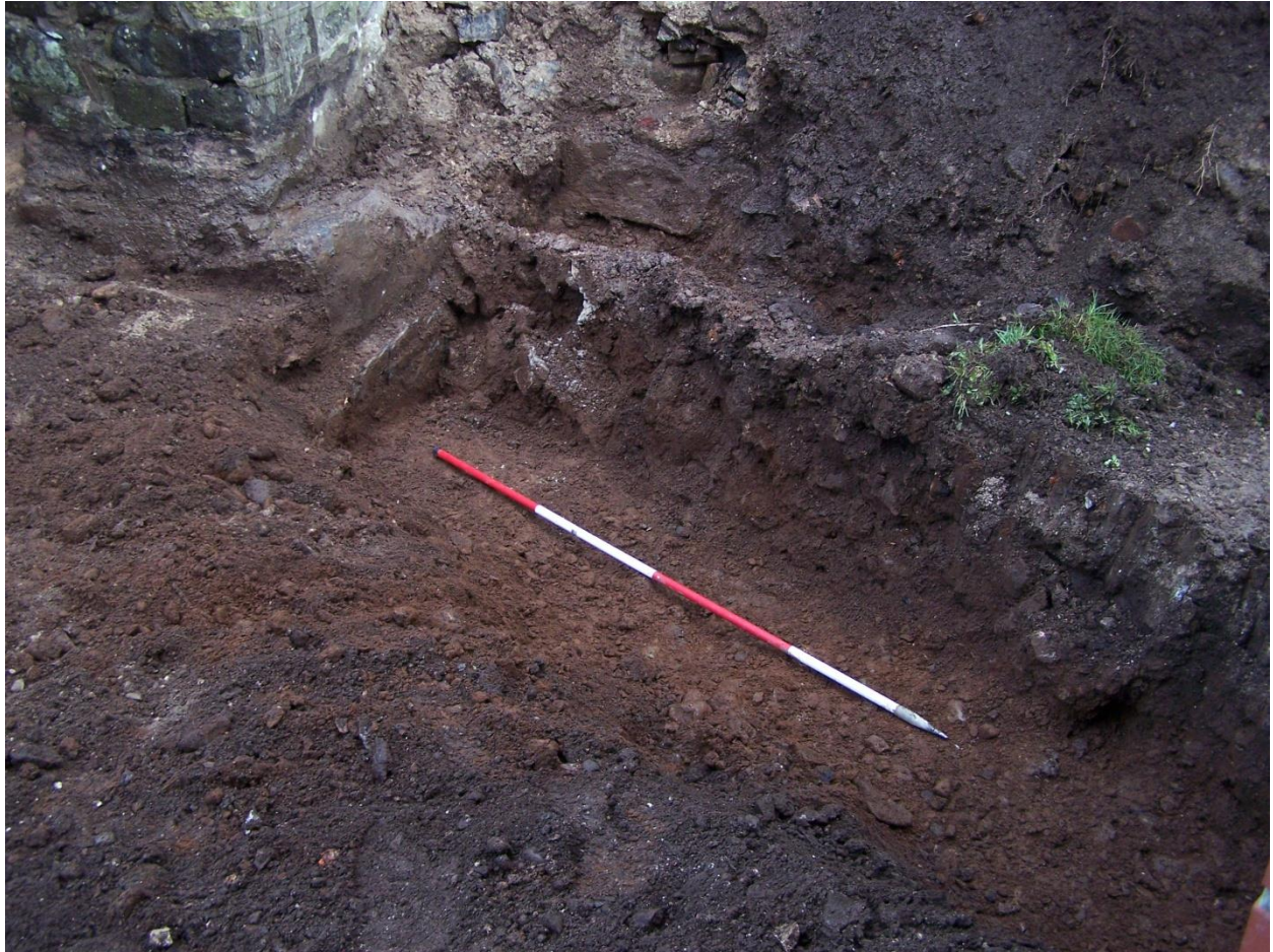
Photo 2: Foundation for east wall of porch (Area 2) after excavation, showing location of removed retaining wall (Area 3) in background.
