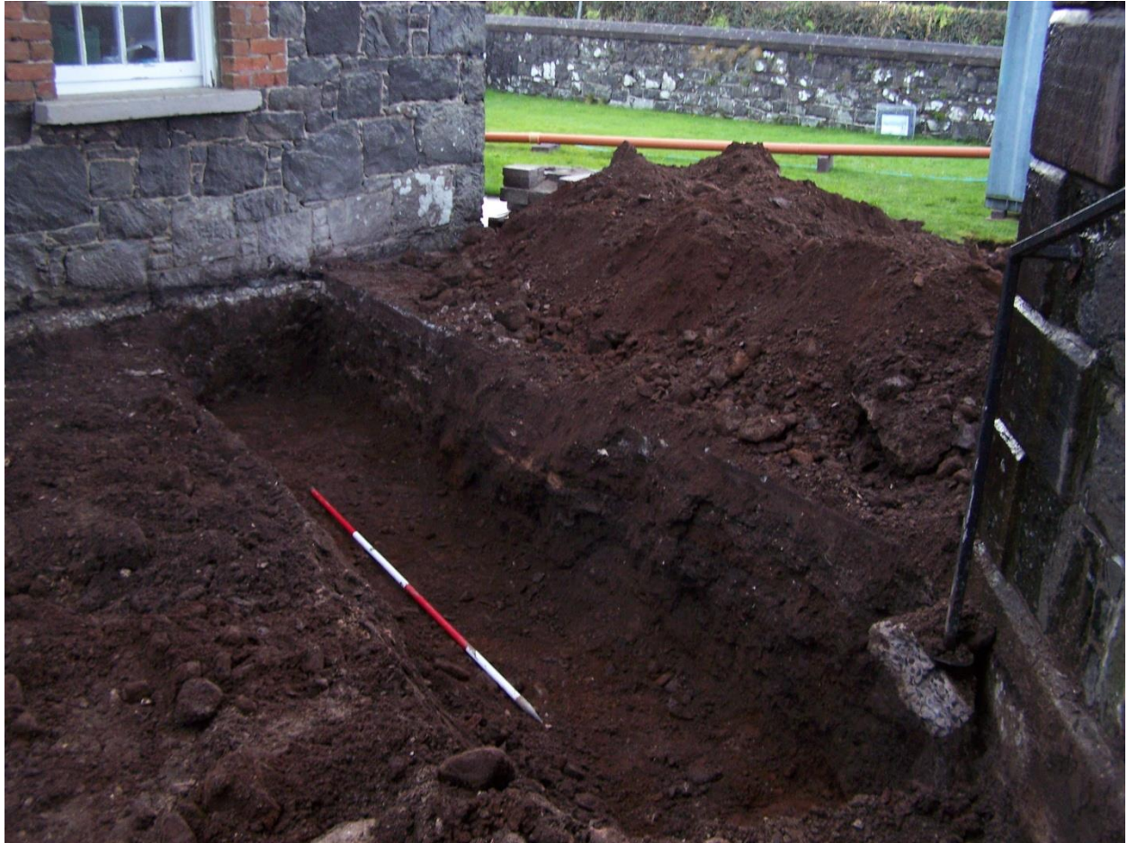
Photo 1: Foundation trench of west wall of porch (Area 1) showing tarmac bedding layers and natural subsoil.
