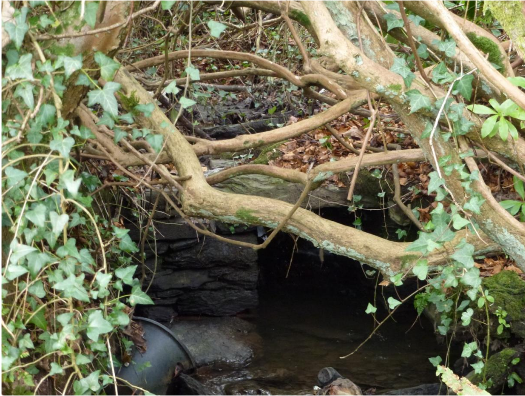
Figure Six: The footings and part of the span of the bridge that crosses the stream close to where it discharges into the Foyle (Irish Grid Reference C45241978). It is possible that this bridge is that depicted upon Nevill's map of the Siege of 1689 and which was probably built by the Jacobite army.
