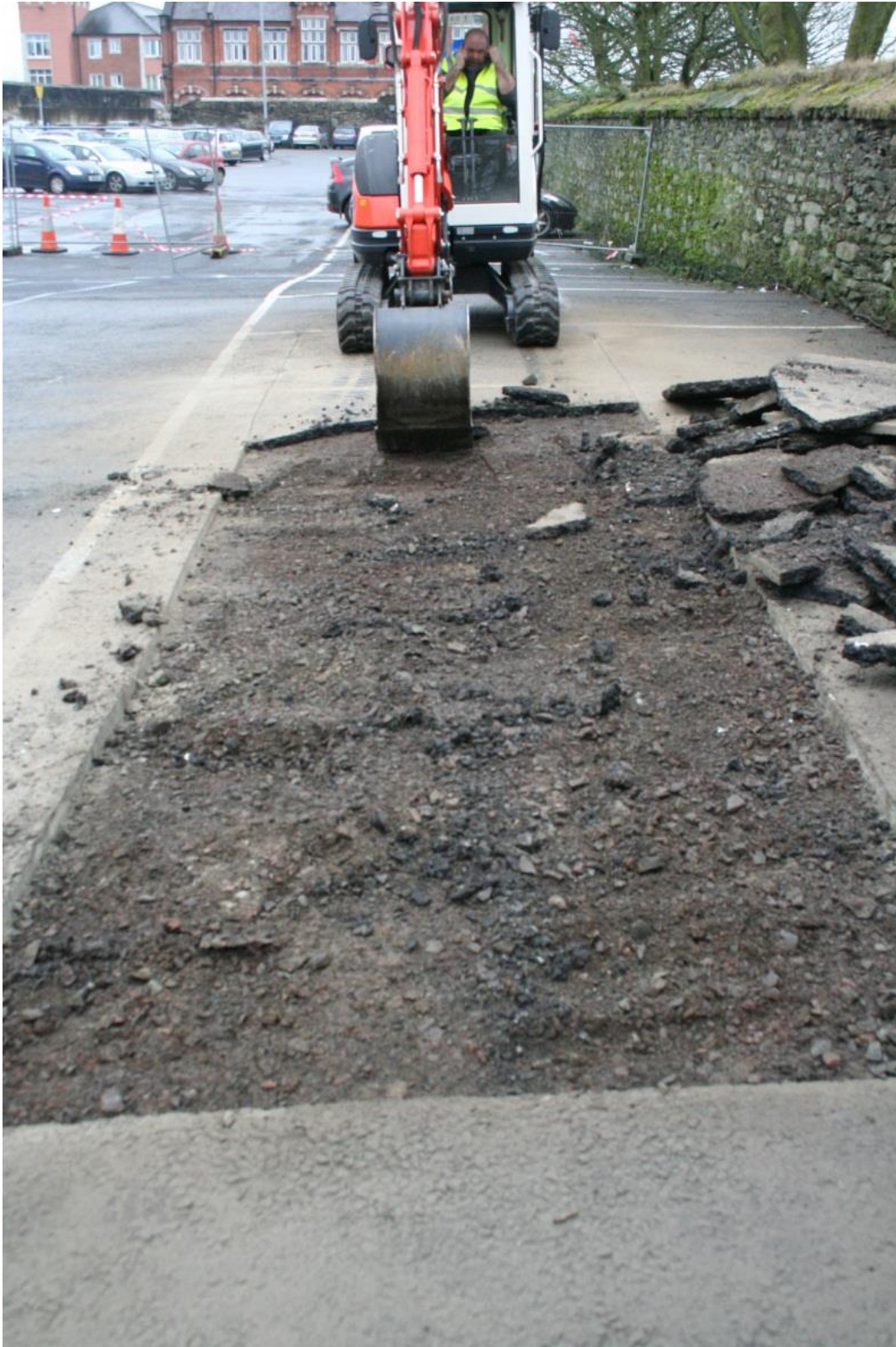
Plate 1 Trench 1: excavation of the tarmac (C101) and quarry gravel (C102) (facing SE).
