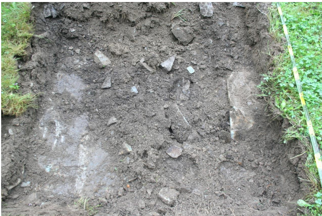
Plate 28: Trench 6, mechanically excavated, showing solid bedrock immediately below the surface, looking SSE
