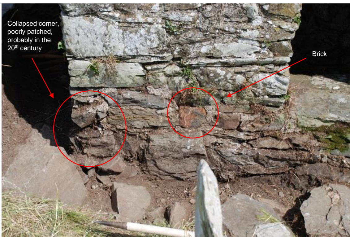
Figure 27 – Brick used in 20 th century repairs to the building, at the south-east corner (above) and in the southern façade (below).
