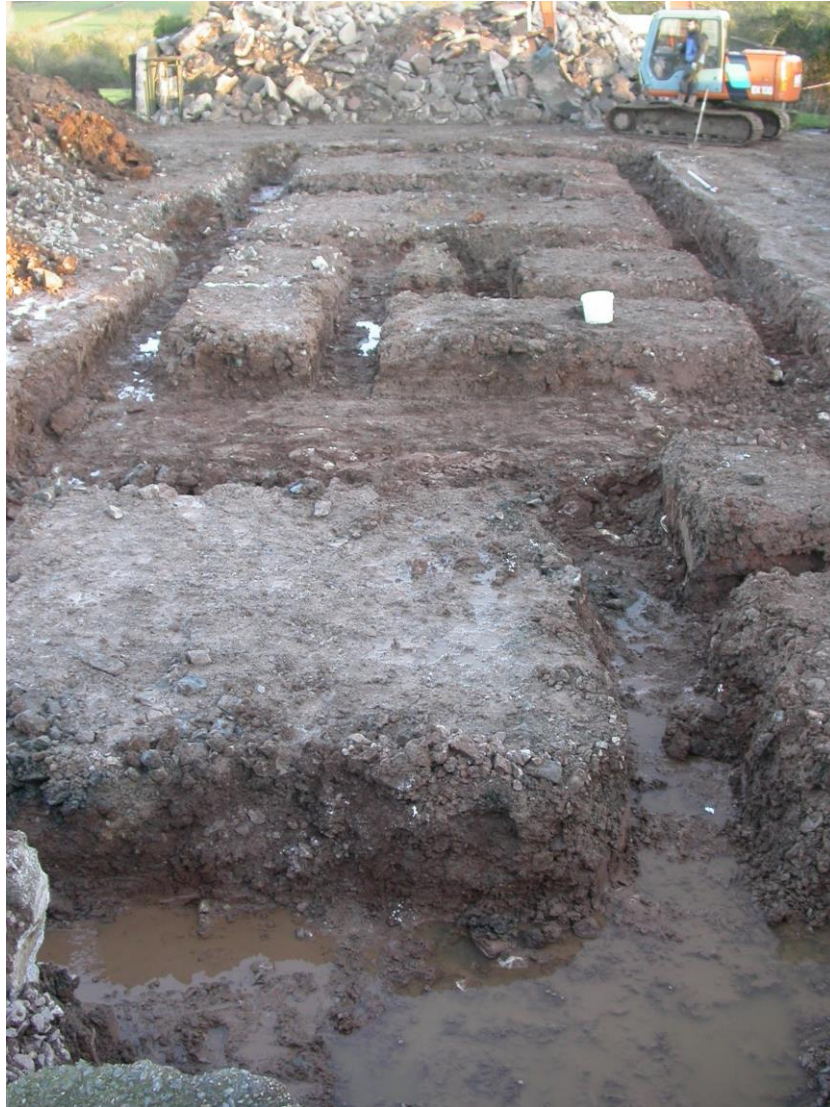
Figure Three: The development site following the excavation of the foundation trenches through the hardcore deposits underlying the removed floor of the demolished barn, looking east (18.1.11).
