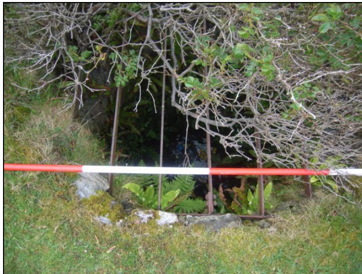
Figure 16: Iron grille at the top of the Lime Kiln flue, Murlough Bay
